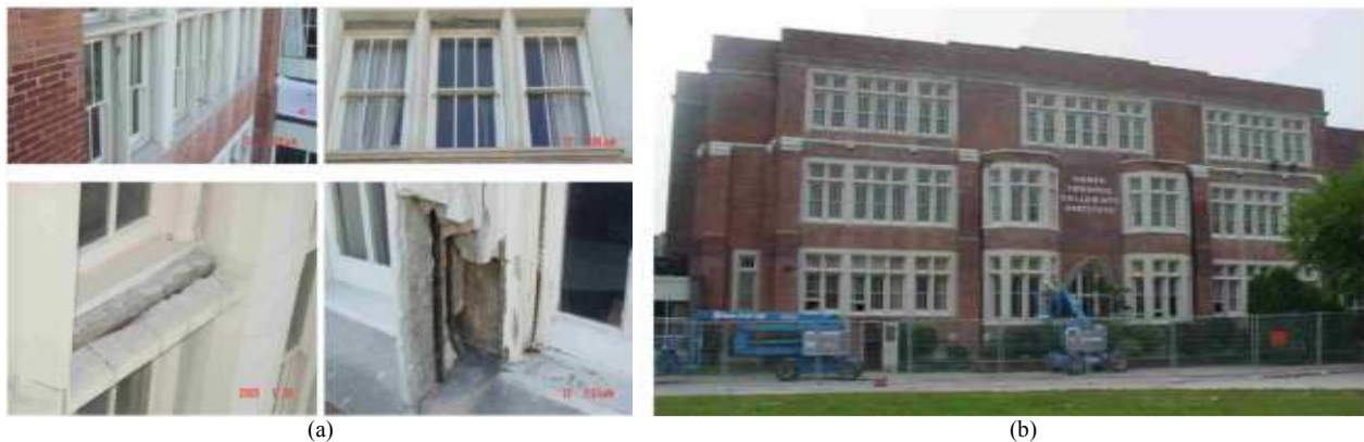
Fig. 4. GFRP retrofitting of a school building in Toronto. (a) example of cracks and severe damage in the (b) overview of the historic building after retrofitting (pictures taken from (Mc Cuaig et al. , 2008))
