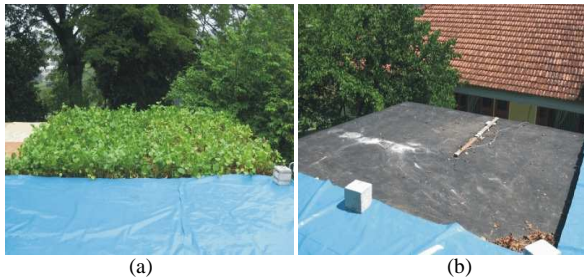
Fig. 3: (a) Roof filled with potted plants (ipomoea pes capre); (b) Bare roof with outdoor surface temperature sensor placed on it surface
