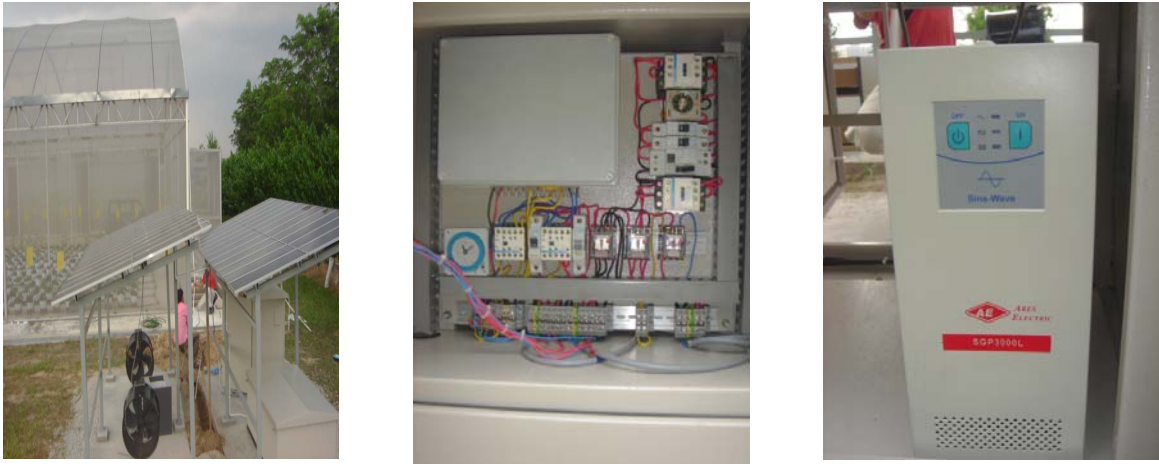
Fig. 2: PV array structure, controller and inverter
