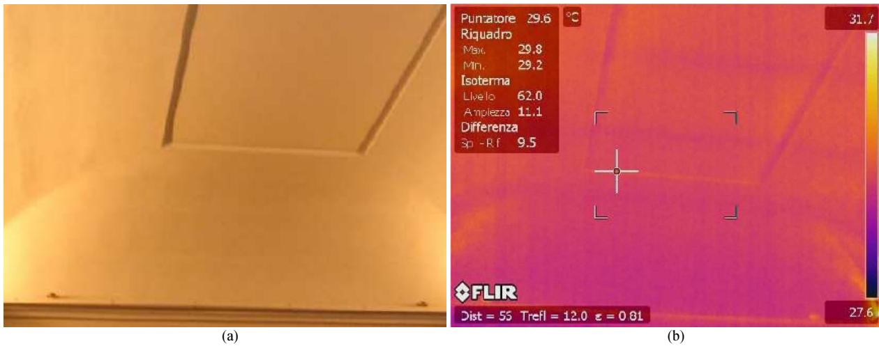
Fig. 5: Room n. 2. (a) view of the intrados of the vault (b) thermographic image showing the timber structure
