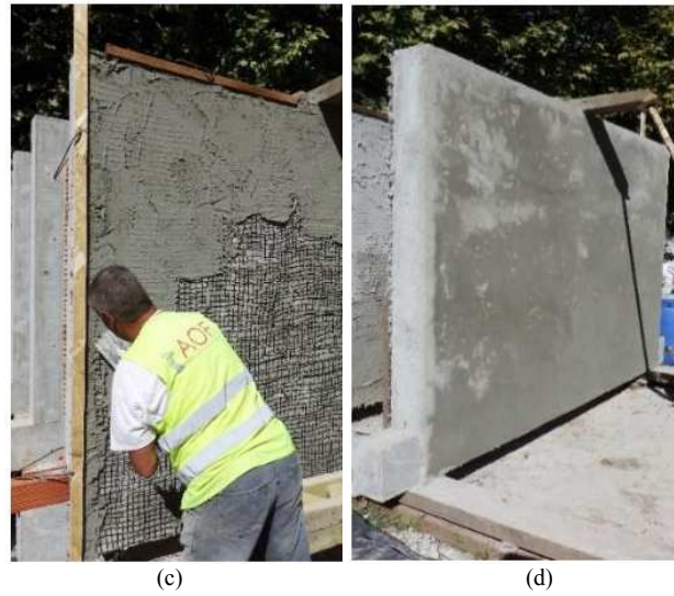
Fig. 5: Application of the reinforced rendering; (a) drilling the pilot holes (b) applying the first layer of mortar (c) positioning of the textile mesh and application of the second layer of mortar; (d) final aspect after rendering
