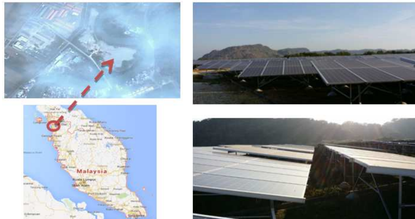
Fig. 2. Solar power plant (Perlis, Malaysia)
