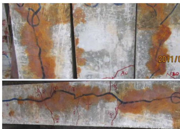
Fig. 6. Corrosion crack map and bending load crack
