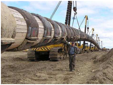
Fig. 1: Building typical ground pipeline. Requires ground right of way and results in damage to ecology
