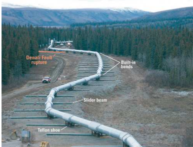
Fig. 2: Trans-Alaska oil pipeline. Notice the damage
