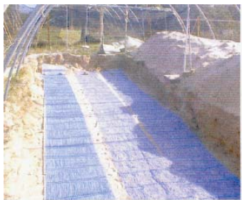
Fig. 2: Capillary heat exchanger buried in the soil of the greenhouse
